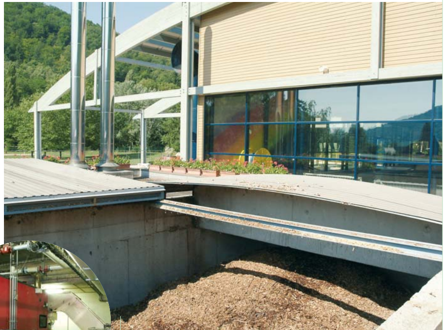
The regions install more and more log heating systems for their public buildings.
